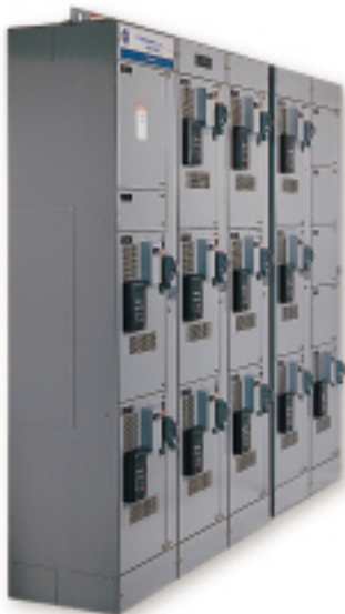
Bulletin 1305 drive units installed in an Allen-Bradley CENTERLINE Motor Control Center.
